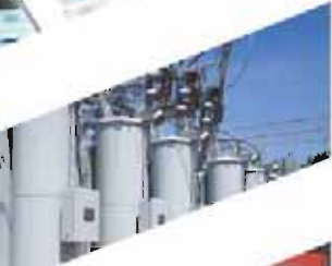
COOPER Power Systems
