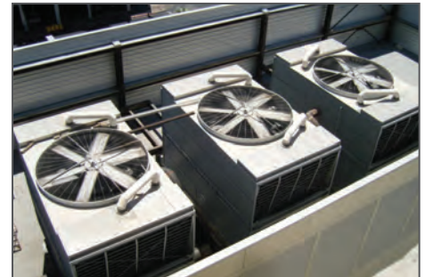
Heating, Ventilation and Air Conditioning (HVAC)
