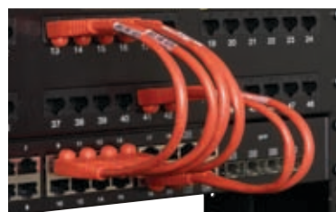
Shown: CAT5e Reduced-Length Cable (EVNSL83-006IN) connecting our GigaBase® CAT5e 48-Port Patch Panel (JPM906A-R5), (p. 161)
