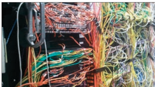
With some time, planning, and SpaceGAIN, you can turn this into a data center showcase. Photo was submitted by a Black Box customer.
