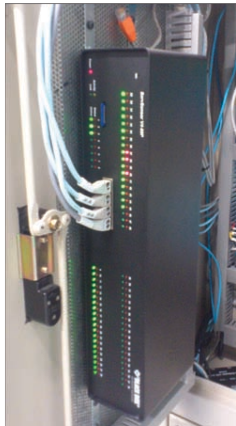
The AlertWerks ServSensor V4E Hub with 60 Dry Contact Inputs (EME134A-60).
