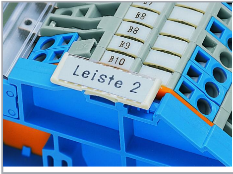
Group marking on N-busbar carrier used as an end stop
