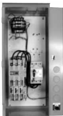
Irrigation Pump Panel
