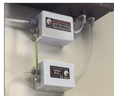
Security alarm panel with ESP TN/BX (bottom) providing protection from transient overvoltages on the dial-up telephone line. Note how the ESP TN/BX is earthed via a bond to the ESP 240-16A/BX (top) installed on the mains power supply to the panel
