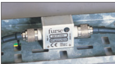
ESP RF 111A11 installed on a coaxial cable running between an antenna and an RF receiver. Note the earth lead (behind the cable tray) attached to the mounting fixture
