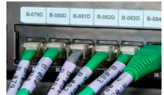
Patch Panel Labels
