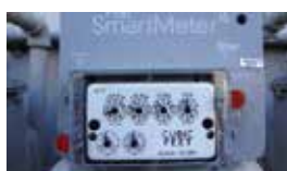
Automated Meter Reading
