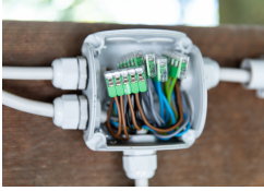
Wiring in the distribution box
