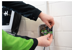
Connection of a wallbox / bicycle charging station
