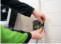
Connection of a wallbox / bicycle charging station
