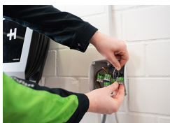
Connection of a wallbox / bicycle charging station
