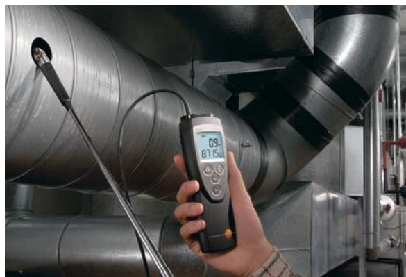
Using the testo 416 to monitor the volume flow of exhaust air
