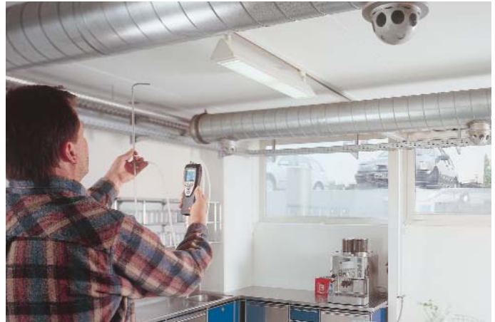
Measuring outlet air
